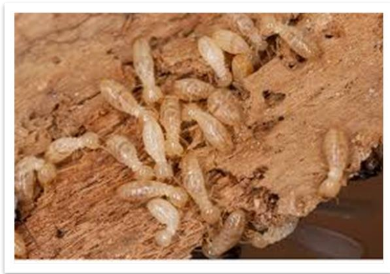
Figure 10. Wood attacked by termites
