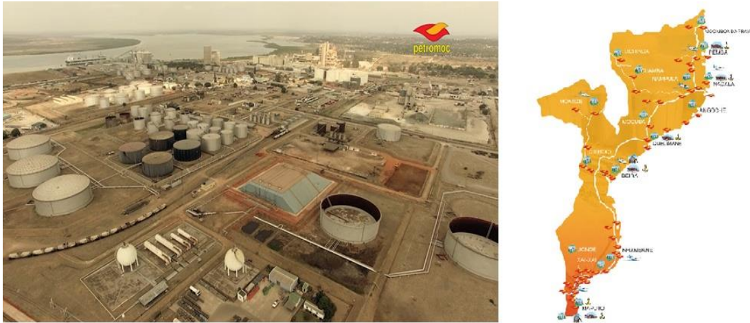
Figure 5: Petromoc's current installation in Matola and its distribution throughout the country (Adapted from company profile 2016).
